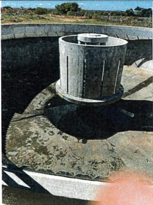
Secondary Settling Tank No.1
