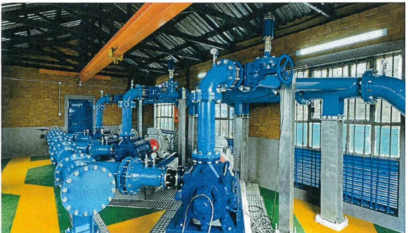
Mabeskraal Bulk water supply Pump Station
