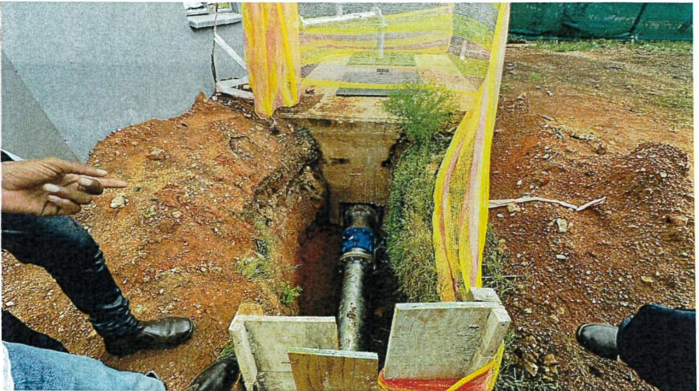
PIPE CONNECTION AT MABESKRAAL WATER PUMP STATION
